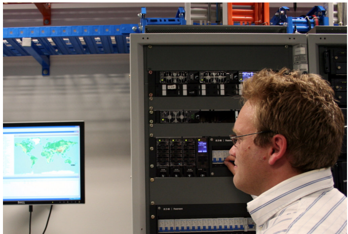
Figure 1: Geoff Callander working with power systems at Eaton
